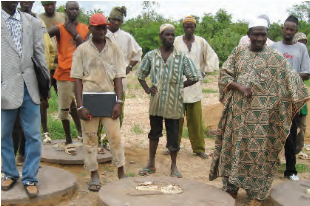
NEW LATRINE CONSTRUCTION: Cement slab production in Socourani, Mali (WAWI partners: SNV and Peace Corps).
